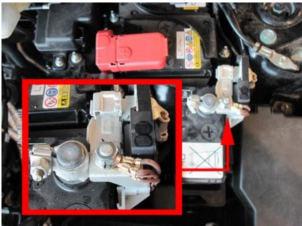
Ground connection on battery.
